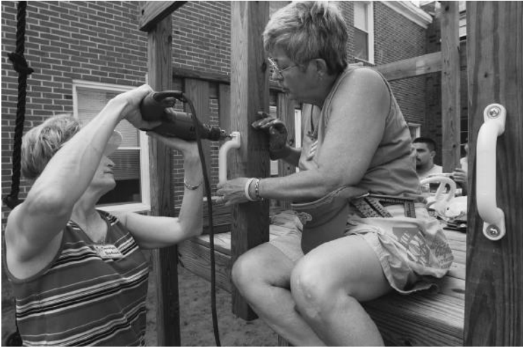
PHOTO 6.2 Volunteers working on installation of a playground after Hurricane Ivan and Tropical Storm Arlene. (Source: Leif Skoogfors/FEMA photo.)
